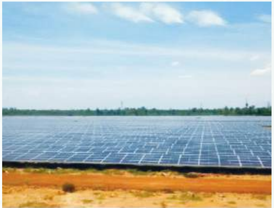
Ground-mounted Solar Power Plant for Captive Consumption by an automobile manufacturer
