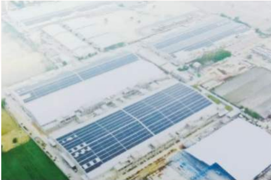
Rooftop Solar Plant for captive consumption by a textile company
