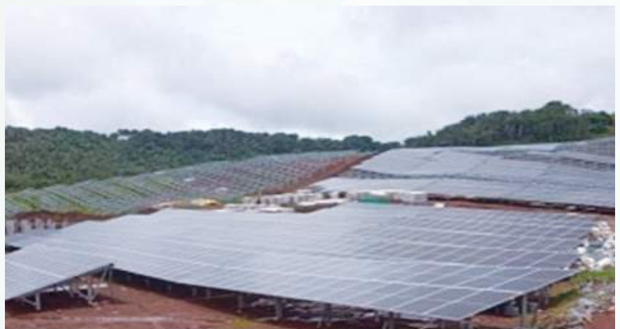
Solar PV farm in Mauritius
